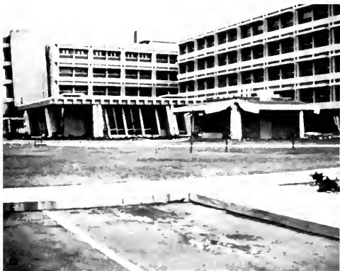
Photo 33. Note partially overturned stair tower at left. Fume Exhaust Building in center right had broken cantilevers (photo 43).
